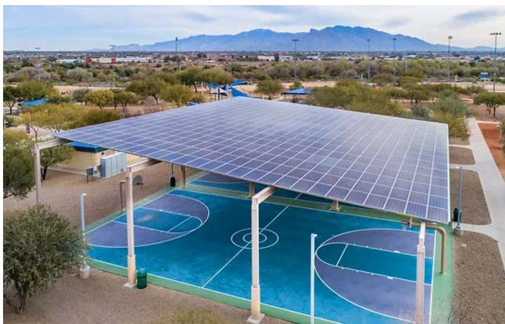
Figure 23. Silverbell Park's basketball solar canopy in Tucson, Arizona.
